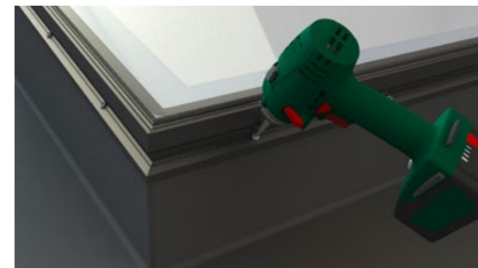
3 Screw the Rooflight onto the kerb using appropriate fixings. Secure it 150mm from the ends and 250mm centres.
